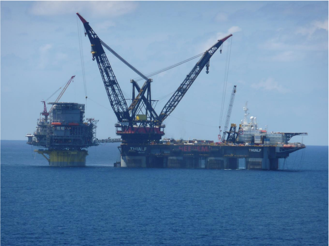
Foto: Wikimedia Commons SSCV Thialf installing the Spar platform Perdido in the Gulf of Mexico
